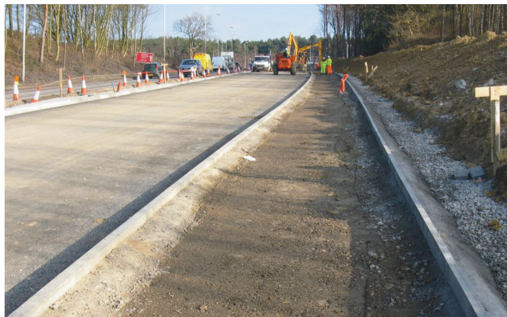
Construction work for North Farm Improvements (Tunbridge Wells), part-funded by the Department for Transport's Local Pinch Point Fund
